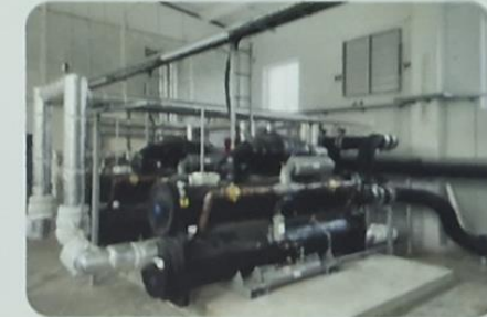
New compression heat pumps 0.6 MW (Jonavos D Company)
